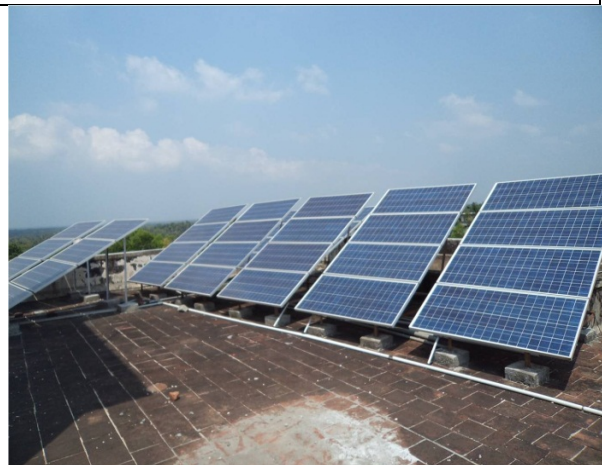
Solar Power System
