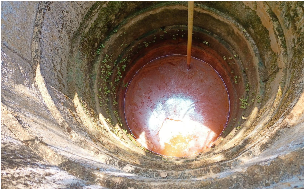
Photo 7: Quality deterioration noted in Thonnakal
